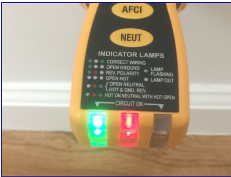
The South side back bedroom has an electrical receptacle on the West wall with reversed neutral and hot.
