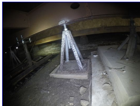
The 12 foot metal jacks under the home are covered with surface rust and should be monitored.
