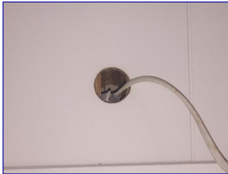
The Master bedroom has an extension cord plugged into a receptacle and running back into the wall for a wall hung TV.
