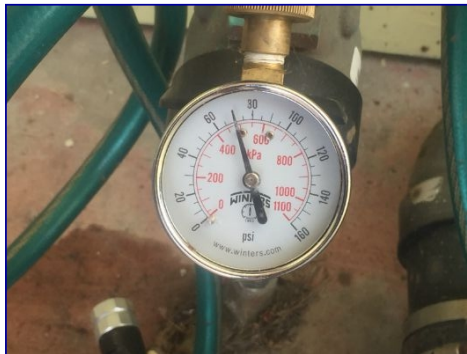
The home's water pressure is 70 PSI.
