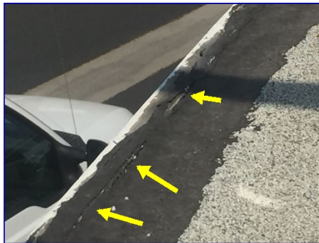
The edges of the roof (front and back) need a new coating of roofing mastic.
