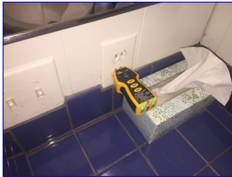
The bathrooms do not have GFCI protection.
