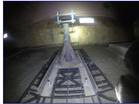
The home has earthquake anchoring jacks installed.
