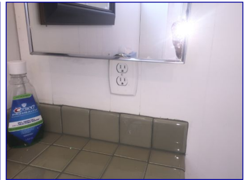
The Master bathroom has no GFCI protection.
