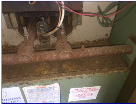
The furnace is heavily rusted inside.
