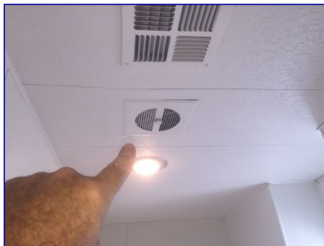
The Master bathroom exhaust fan is noisy.
