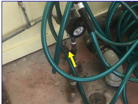
The home's main water shutoff is in the carport area.
