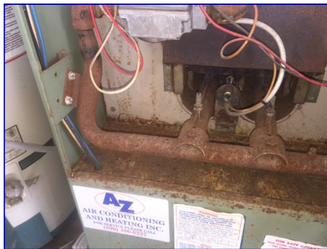
The furnace is heavily rusted inside.
