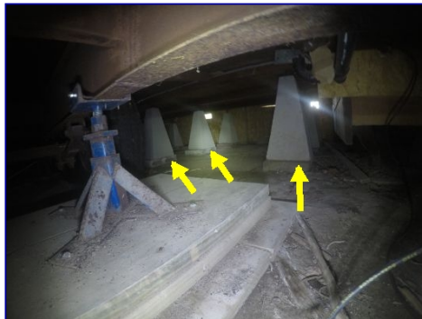
The front porch area of the home has concrete piers installed as supports.
