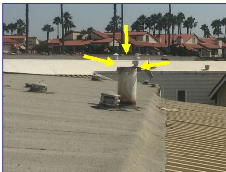
The furnace exhaust pipe on the roof is missing a cap.
