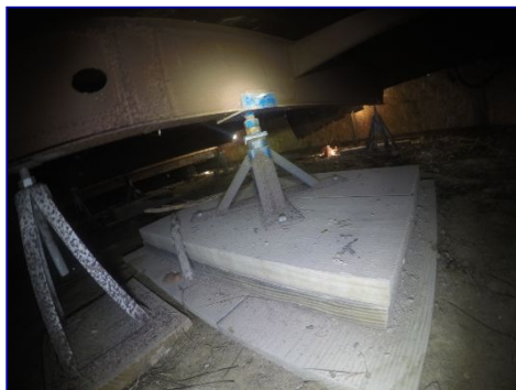
The home has earthquake anchoring jacks installed.
